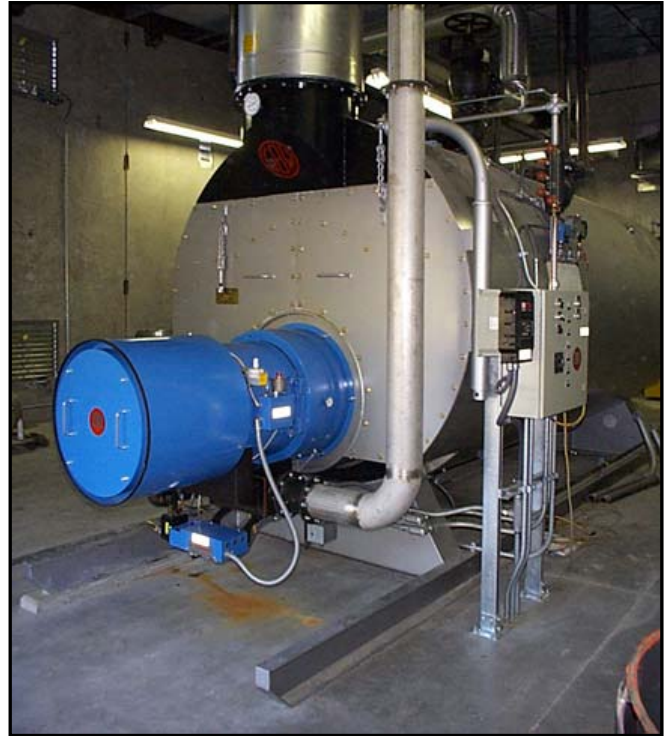
300 HP firetube boiler application
