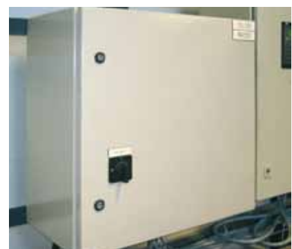
Panel de control OK100
